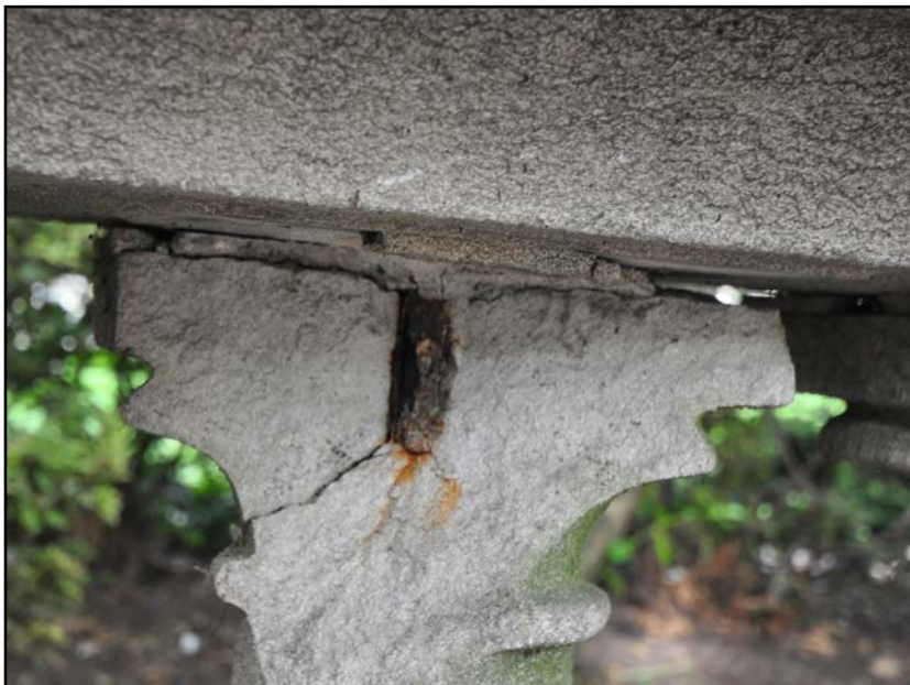
Figure 2: Spalled stone due to rust jacking at a balustrade at Rittenhouse Square in Philadelphia, PA. Credit: Brian Rich, 2013
