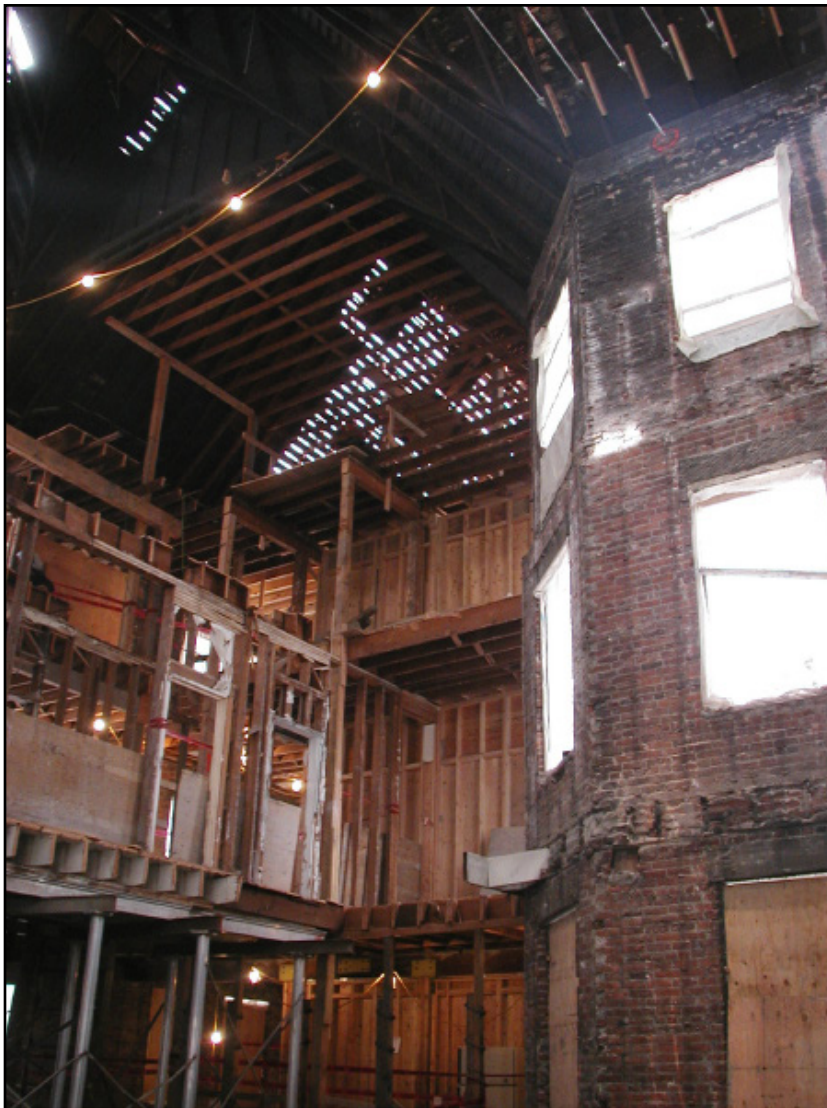
Figure 14: Clark Hall interior during demolition showing the removal of major portions of the interior construction. View looking north. Credit: Staff photo courtesy of UW CPD, June 2008.
