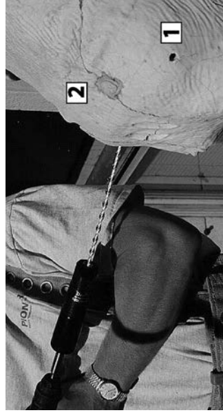
Fig. 7. 1996 walrus head rehabilitation. Note the drilled hole (1) for insertion of a helical anchor to pin sections of the walrus snout that had fractured due to expansive grout in the cavities of the terra cotta unit. The white dot (2) on top of the nostril is where the expansive grout was injected in the 1982 repair. (Credit: Wiss, Janney, Elstner Associates, Inc.)
