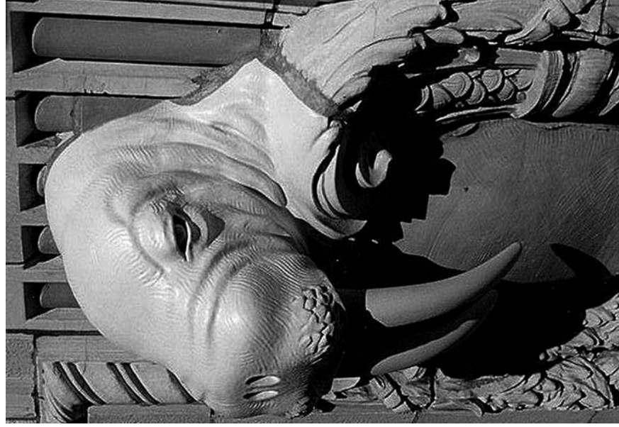
Fig. 8. 1996 replica walrus head. The joints between terra cotta pieces are filled with mortar after the epoxy sets around the threaded rod anchors. (Credit: Wiss, Janney, Elstner Associates, Inc.)
