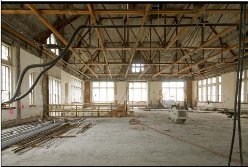
Figure 25: The 2009 renovation retained the structure and historic shell of Savery Hall. Credit: John Stamets, 2008, courtesy UW CPD.
