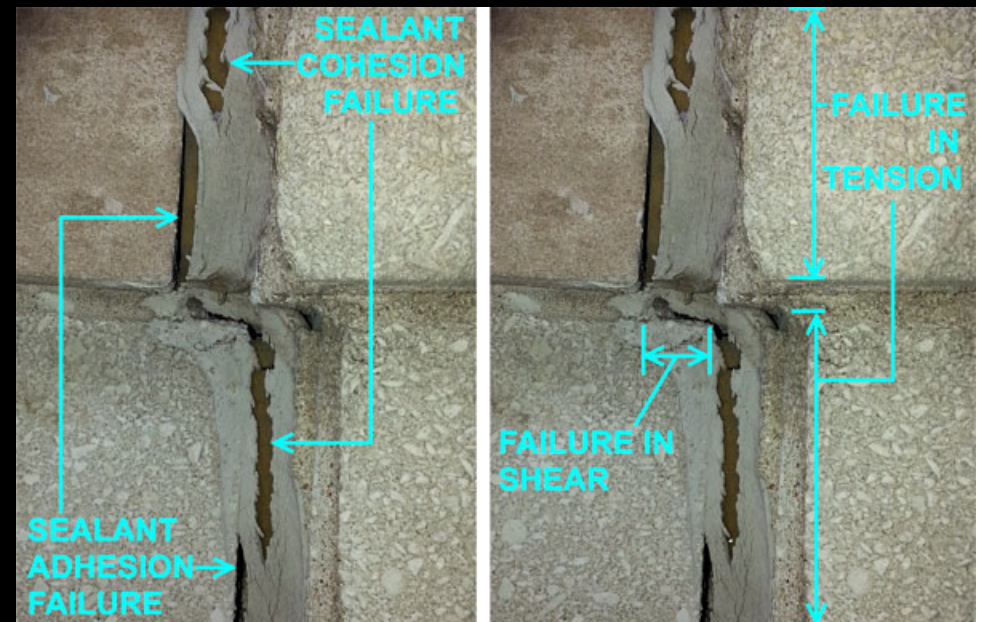
Figure __: Modern sealants fail due to the adhesion to surfaces or internal cohesion of the sealant. Credit: wikimedia
