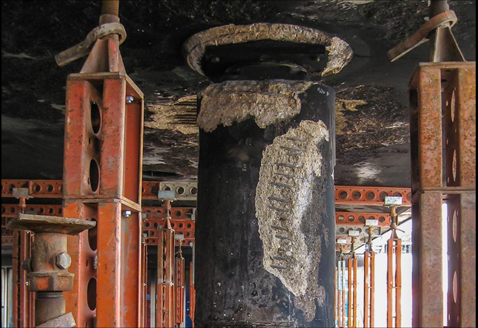
Figure __: Fire damaged concrete can spall, exposing rebar to corrosion and even melting rebar in sustained fires. Credit: www.sandberg.co.uk , 2014
