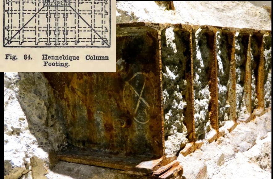
Figure __: Foundations often have crossing layers of steel beams (top left, credit: Hennebique-Radford's cyclopedia of construction, 1909) forming a "grillage," as at the south tower of World Trade Center (bottom right, credit: howdoyoumeasure525600minutes.com, 2001)
