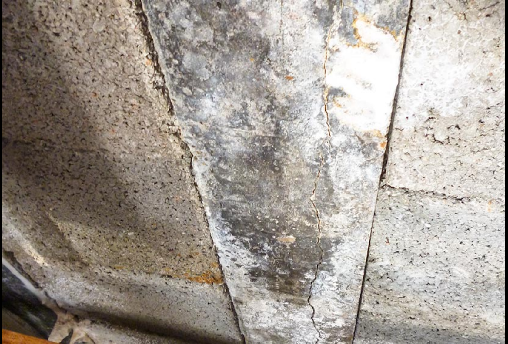
Figure __: High alumina cement deterioration is caused by reactions of the alumina to other components of the concrete leaving voids that become structurally weak points in this concrete joist. Credit: www.sandberg.co.uk , 2014
