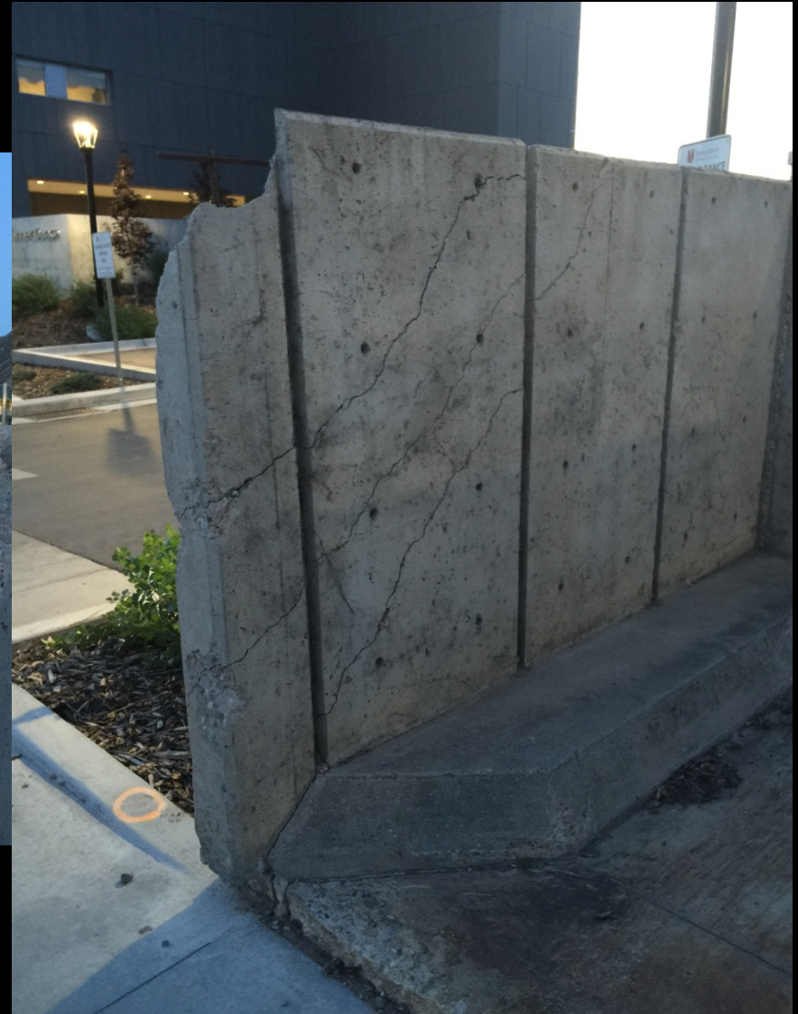
Figure __: Concrete deterioration isn't just chemical or corrosion based. It can also be mechanical, such as this damage by a garbage truck that ran into the concrete wall. Credit: Brian Rich, 2015.
