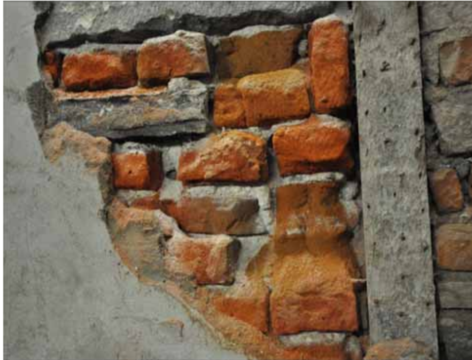
Figure 3: Deteriorating brick, mortar and plaster at the barracks at La Citadelle de Quebec. Credit: Brian Rich, 2014
