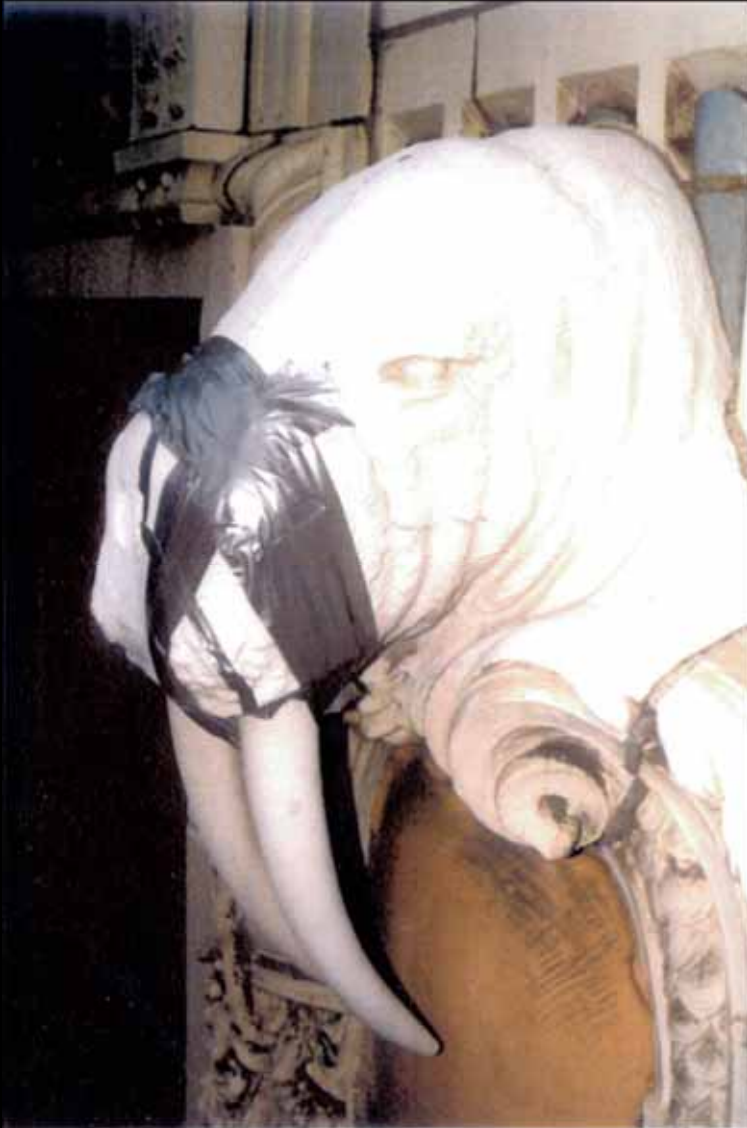
Figure 47: 1995 photo of the deteriorated walrus head at the Arctic Building. Credit: Wiss, Janney, Elstner, 1995.
