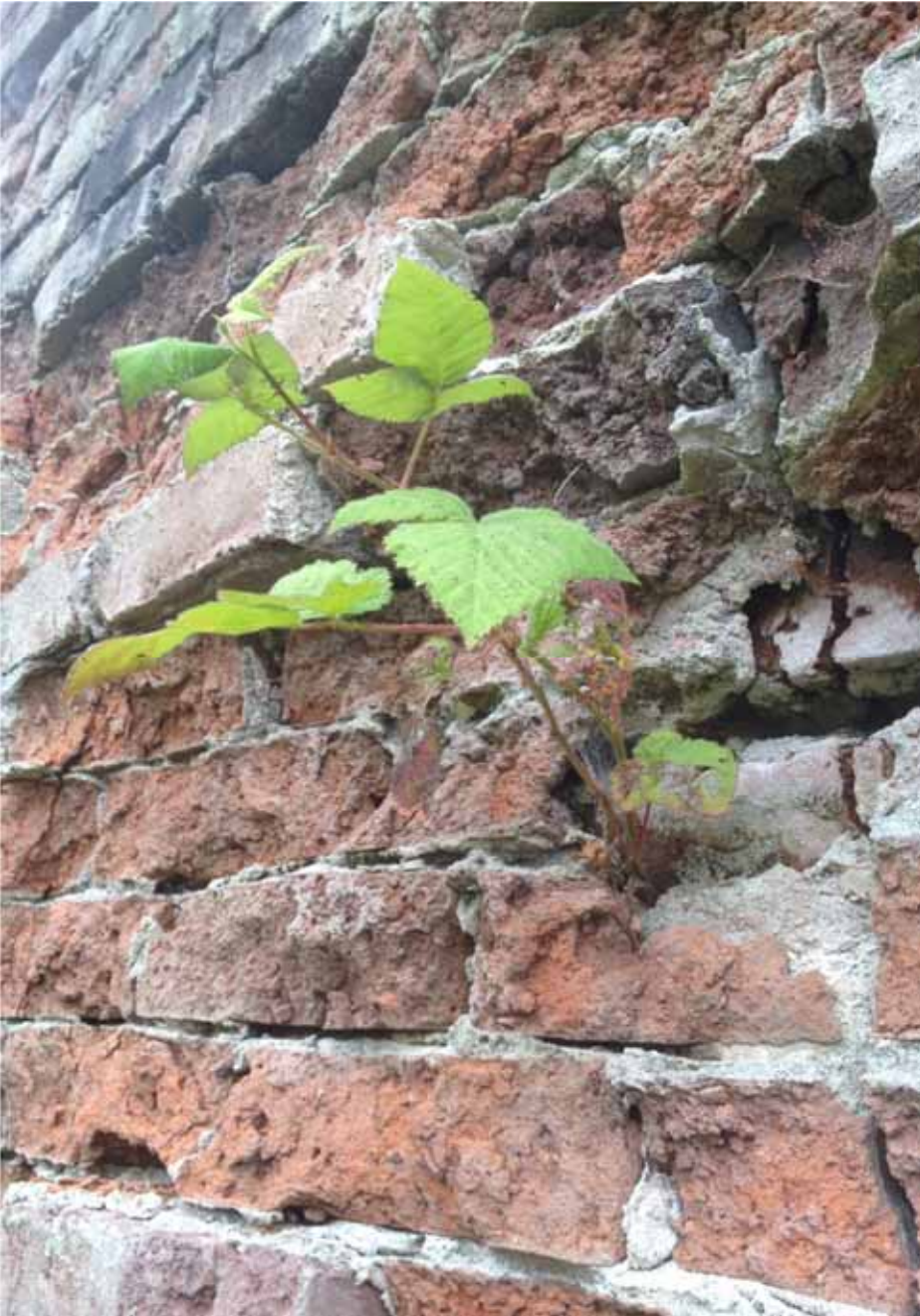
Figure 0: Brick and mortar deterioration at an exterior site wall. Credit: Brian Rich, 2013
