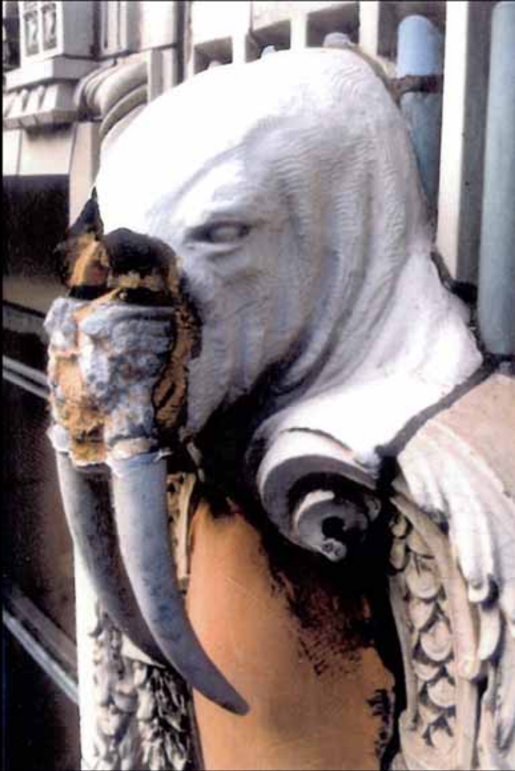
Figure 48: 1995 photo of the deteriorated walrus head at the Arctic Building. Credit: Wiss, Janney, Elstner, 1995.
